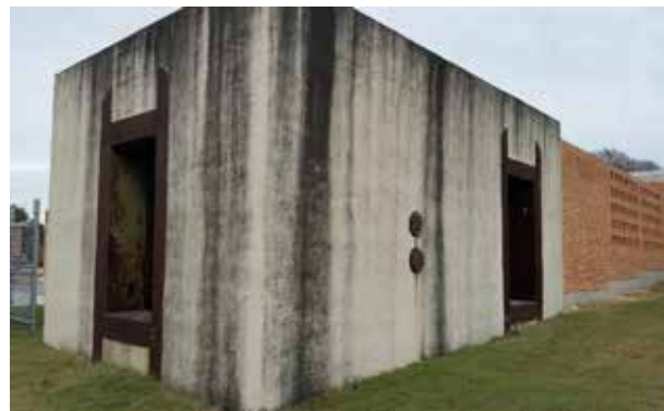
Figure 3. The concrete chamber in a state of abandonment. Courtesy WT Workman.
